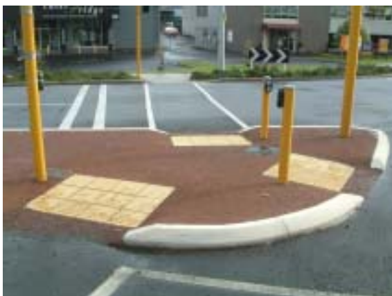
Photo 14: Warning indicators correctly installed on this slip lane island, in regard to alignment and position. Cutting the island through level with the roadway would improve guidance across the island and accessibility for mobility-impaired people. In the absence of the cut-through directional TGSi should be considered. Also note how exclusive pedestrian push button poles have been provided adjacent to each crossing point (refer Section 5.5 for guidance).
