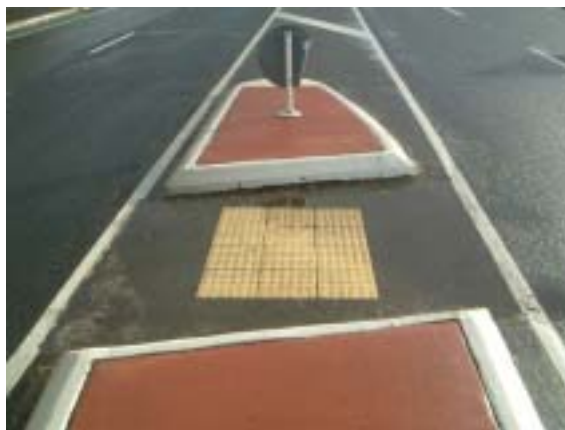
Photo 9: Warning indicators correctly installed across the full depth of this pedestrian median island (1.2-1.8m deep). Note: Warning indicators should cover full width of cut through. This one could be bypassed.
