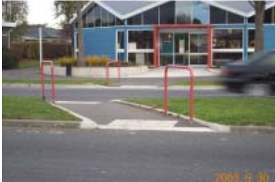
Photo 10: On deep medians two sets of warning indicators are installed. (Note: not quite full width.)
