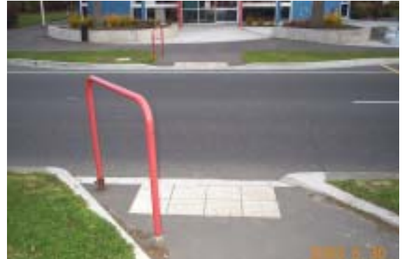
Photo 11: The warning indicators are aligned with the road crossing direction. (Note: not quite full width.)
