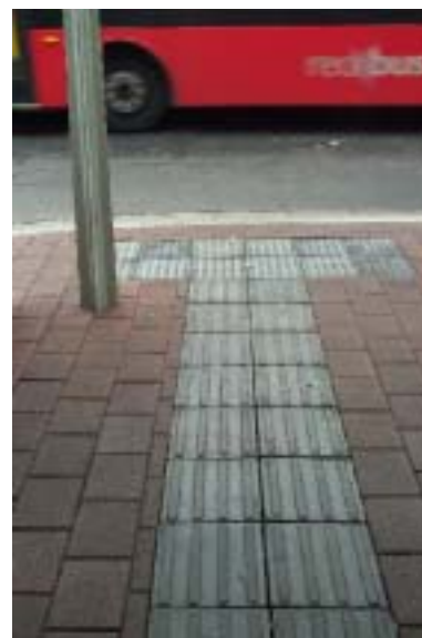
Photo 17: Directional indicators lead to warning indicators at a bus stop. Note the warning indicators are wider than required.
