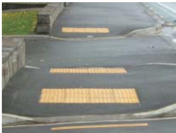
Photo 12: Warning indicators should be installed at all intersections, no matter how minor.
