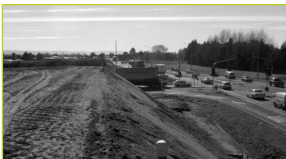
Improvements at the intersection of the Meanee Road interchange with the Hawkes Bay expressway on SH 50, near Taradale, will ease traffic congestion and improve safety. Photo courtesy of Transit.
